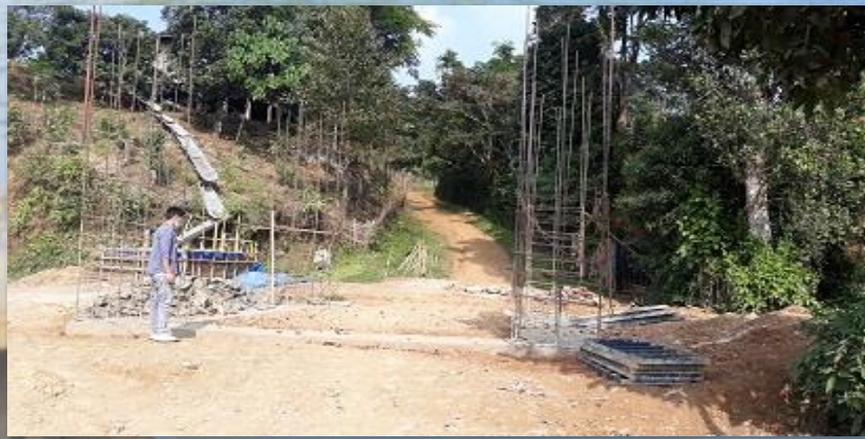
DMU Longleng: ADMU Head along with department staff visited Kangching village to check the progress of village gate construction (EPA) as well as the JAF model Kangching
