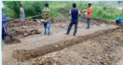
Construction of Marketing Shed cum water collection tank (WHS) at Piphema Old Village (Batch-II)
