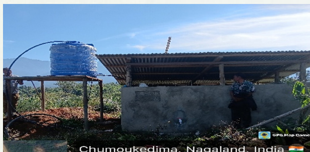
Drinking water filter installed under WHS at Ruzaphema Village, DMU Dimapur
