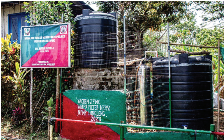
Water Filtration Plant installed at Yachem village
