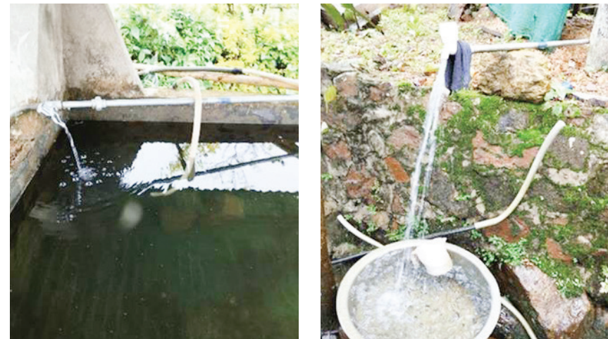
Water Collected at the WHS through Pipelines
